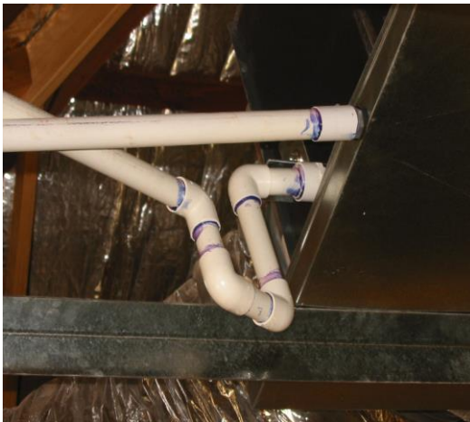
MAIN DRAIN AND EMERGENCY DRAIN
